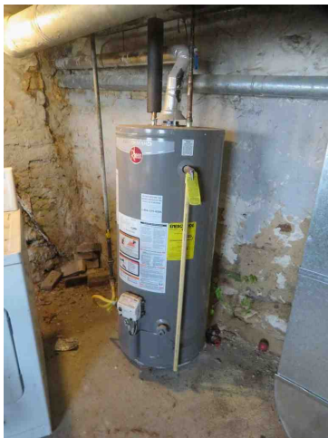
Hot water heater
